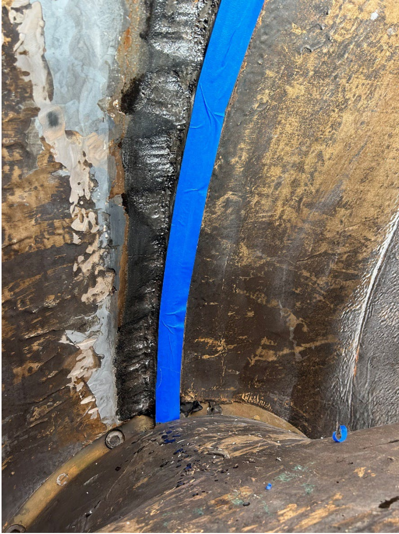
Figure 3.—Power tool cleaning to metal of the cavitation damage downstream of the butterfly seat. The blue tape is protecting the stainless steel seat. The 3/8-inch-deep cavitation damage is to the left of the tape.
