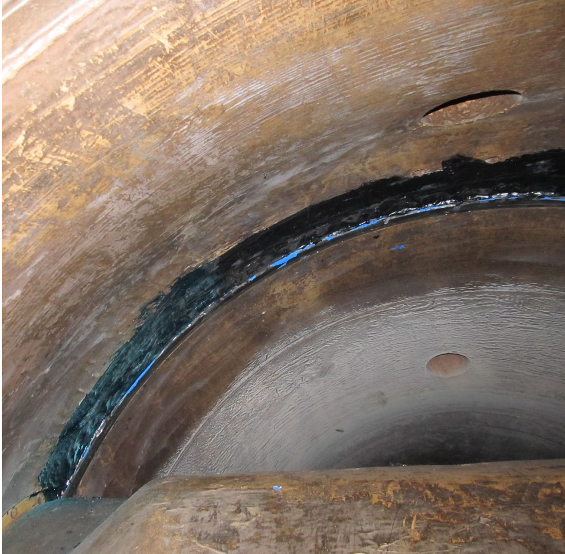
Figure 11.—Test area is shown prior to recommissioning Unit 2 penstocks. Drips and sags had been smoothed, but a few areas still needed to be sanded down to allow for proper operation of the butterfly valve.
