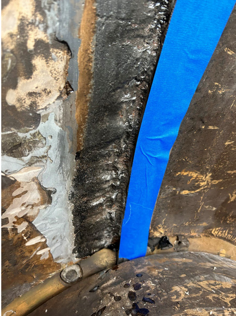
Figure 4.—Powertool cleaning to metal of the cavitation damage downstream of the butterfly seat. The blue tape is protecting the stainless steel seat. The 3/8-inch-deep cavitation damage is to the left of the tape.
