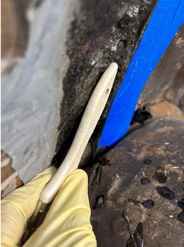
Figure 5.—Cavitation damage downstream of the butterfly seat shown after power tool cleaning exposed pits up to 3/8 inches deep.
