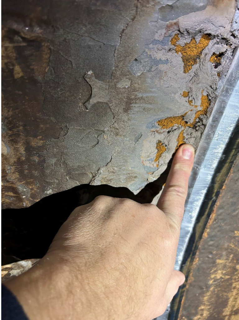
Figure 2.—Condition of the cavitation damage downstream of the butterfly seat prior to surface preparation.
