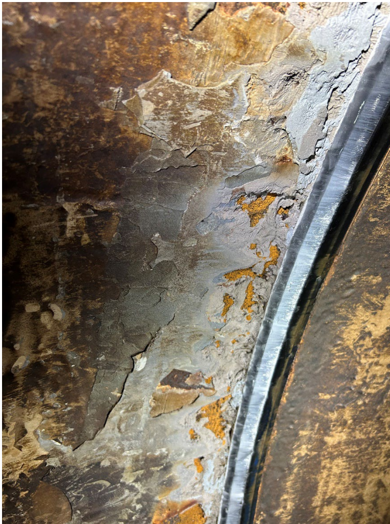
Figure 1.—Condition of the cavitation damage downstream of the butterfly seat (left side of stainless steel seal) prior to surface preparation.
